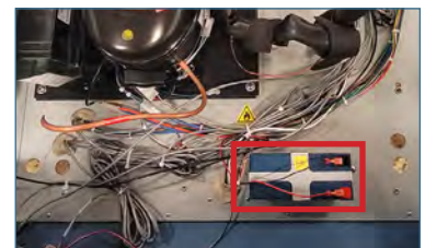
Monitoring system back-up battery.
