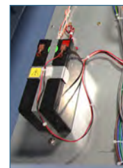
Monitoring system backup battery.
