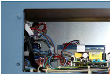
Monitoring system back-up battery.
