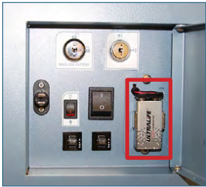
Monitoring system back-up battery.
