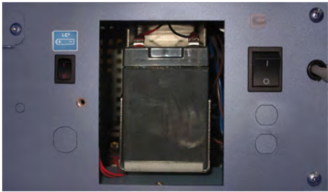
Monitoring system back-up battery.
