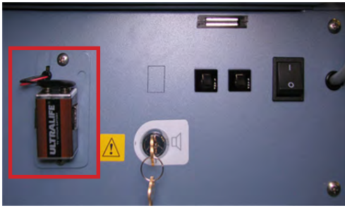
Monitoring System back-up battery.
