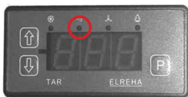
Independent temperature controller (defrost lamp circled).
