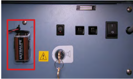
Monitoring system back-up battery.
