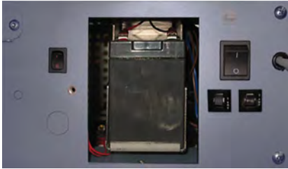
Monitoring system back-up battery.
