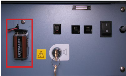
Monitoring system back-up battery.
