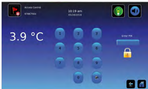
Access Control keypad
