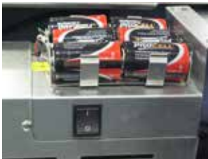
Monitoring system backup batteries.
