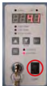
Light switch (circled).
